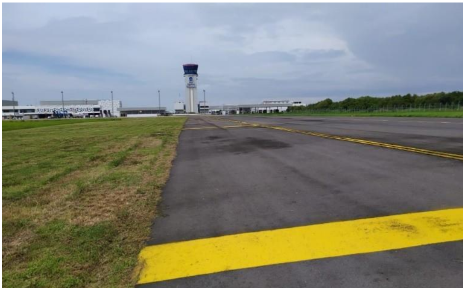
Penurunan \pm 6,5 cm taxiway shoulder F
