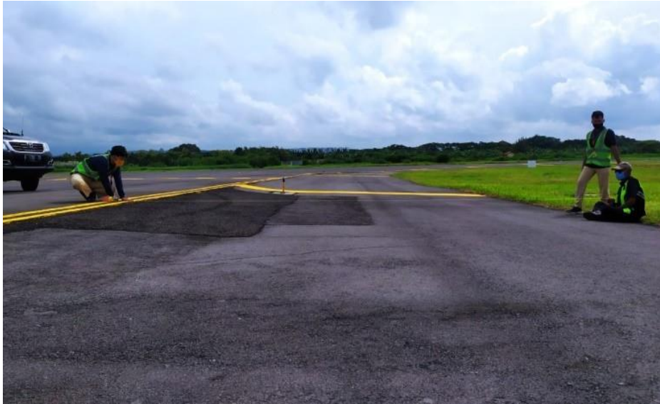
Penurunan \pm 23,75 cm taxiway shoulder G
