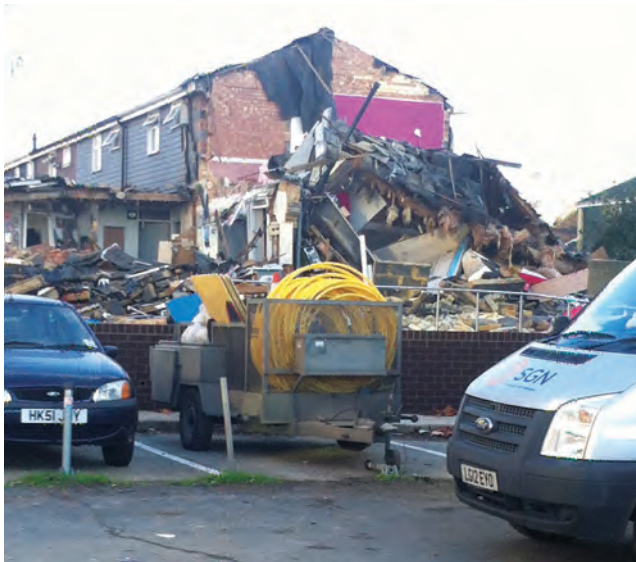
Figure 16.10 Gas explosion during the night but man and his daughter escaped unharmed – house destroyed, Southampton, 2014
