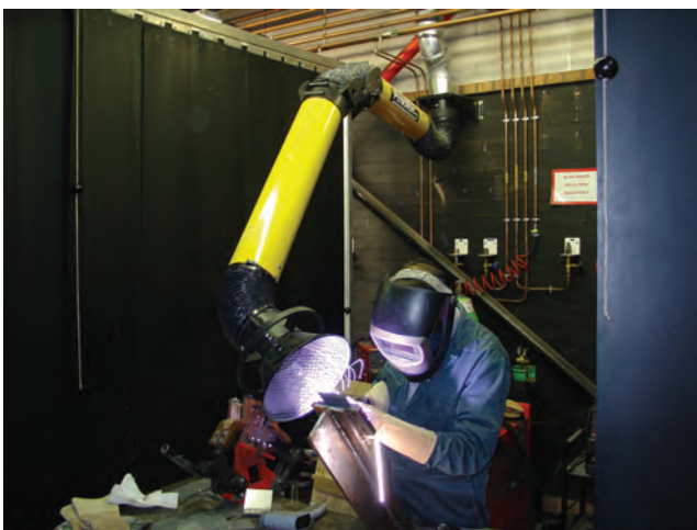
Figure 13.12 (a) A LEV system; (b) welding with an adjustable LEV system to remove dust and fumes
