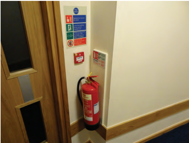
Figure 12.20 Typical fire point in offices with extinguishers, fire notices and alarm break-glass call point
