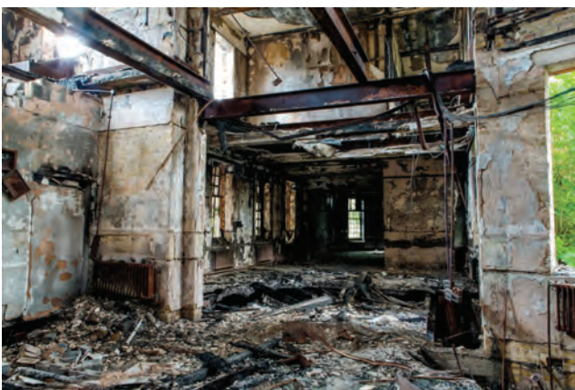
Figure 5.4 A dangerous occurrence – fire
