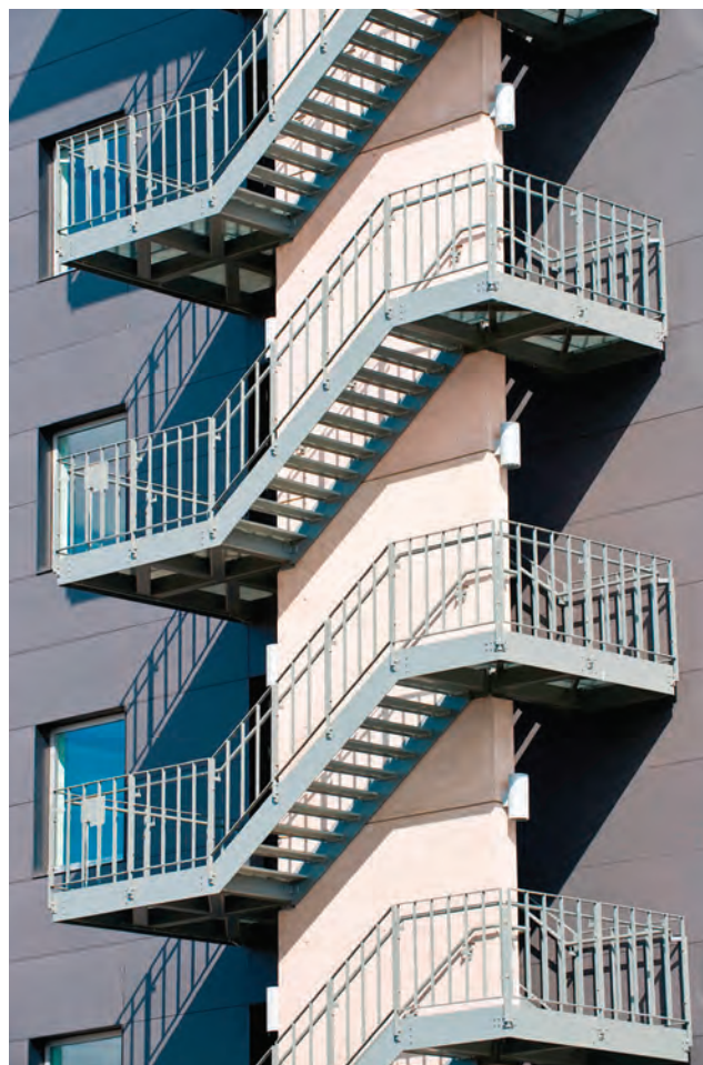
Figure 12.24 External fire escape from a multi-storey building. Extreme caution needed in winter and enclosure of staircase would be preferred for the UK climate
