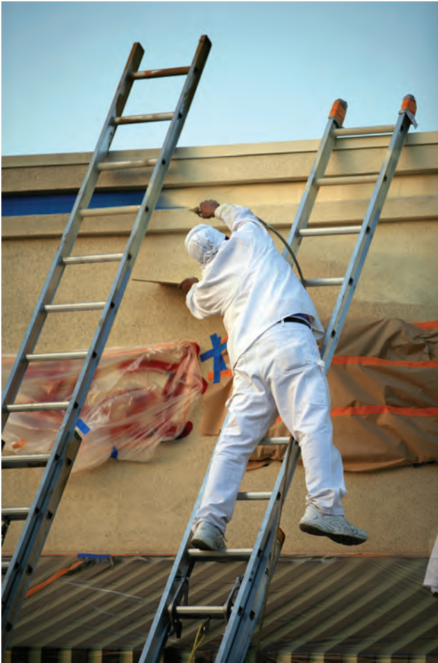
Figure 2.8 The policy might be good but is it put into practice – unsafe use of a ladder
