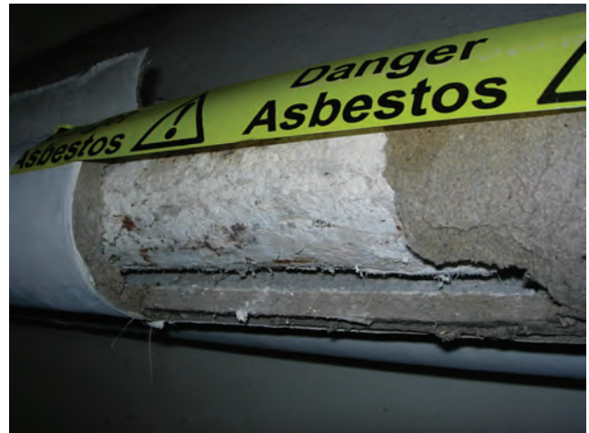
Figure 13.17 Damaged asbestos lagging on pipework
