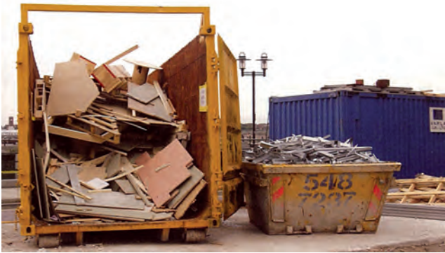
Figure 13.21 A designated waste collection area with two types of skip commonly used for waste collection. Heavy materials would be transported in the smaller skip. Sizes of skip range from about 4 cu metres (small skip shown) to about 35 cu metres (large skip shown)
