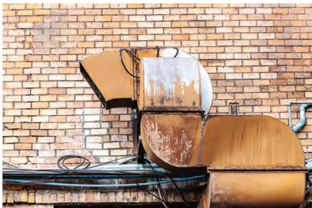
Figure 13.13(a) Local exhaust ventilation systems can quickly corrode and need regular maintenance of fans and filters
