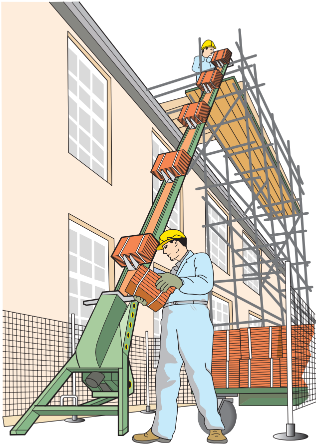
Figure 9.12 A brick elevator
