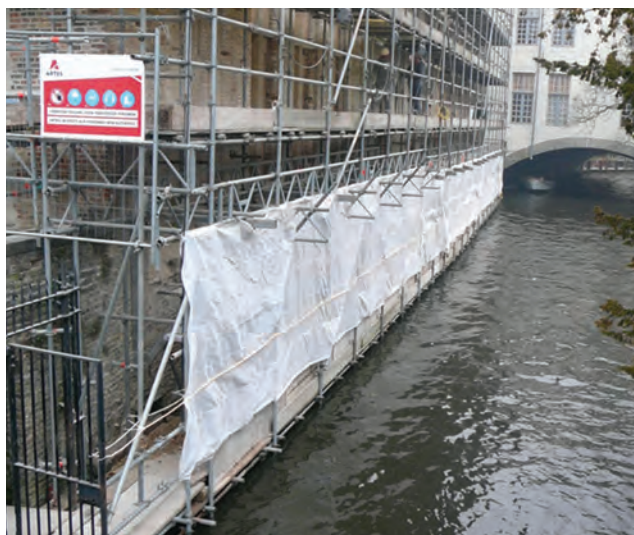
Figure 7.22 Working near or over water – large scaffold with protection screens and a small boat moored under the bridge in case rescue is needed
