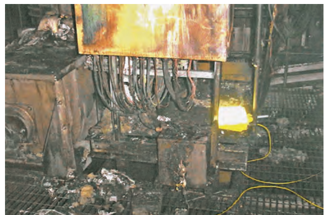
Figure 11.4 Over 25% of fires are caused by electrical malfunction
