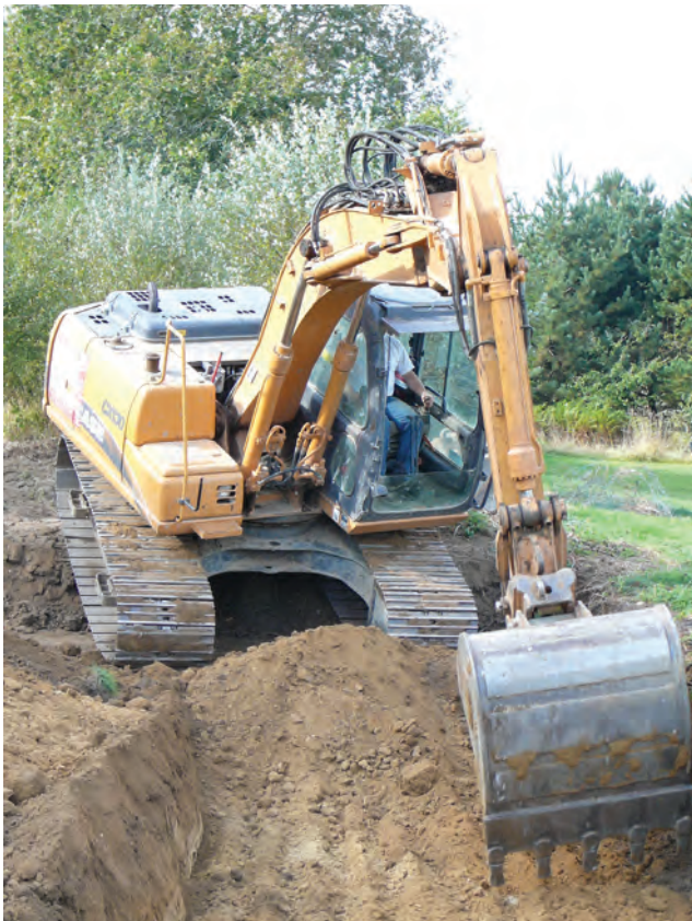
Figure 8.4 Operating a piece of mobile work equipment, an excavator, to excavate a swimming pool
