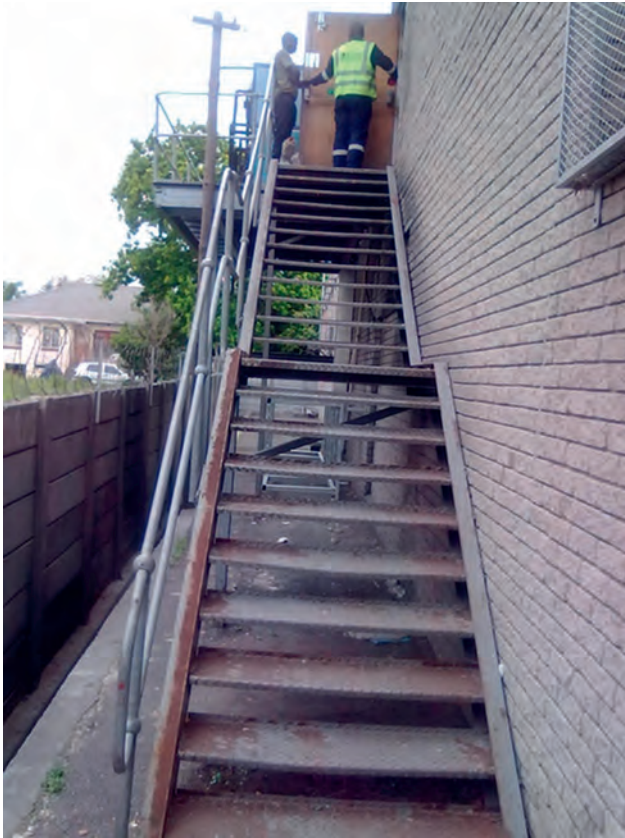
Figure 12.25 Fire escape route outside building
