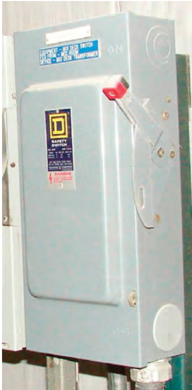
Figure 11.9 A variety of electrical equipment: (a) electrical cabinet with multi-hasps and lock-off padlocks on the isolator; (b) 240 volt socket with RCD devices built in; (c) lockable electrical control cabinet
