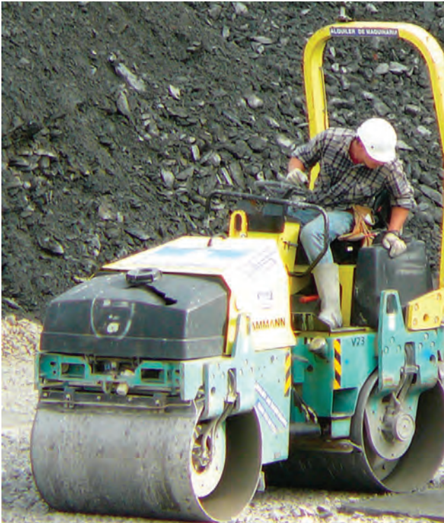
Figure 14.7 (a) Vibrating roller with risk of whole-body vibration
