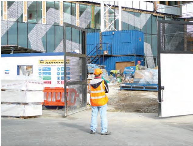
Figure 7.21 Secure site access gates
