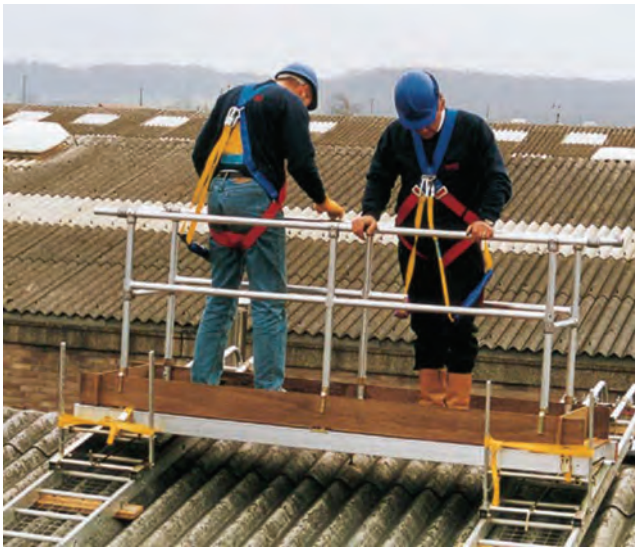
Figure 7.12 Proper precautions must always be taken when working on or near fragile roofs or surfaces
