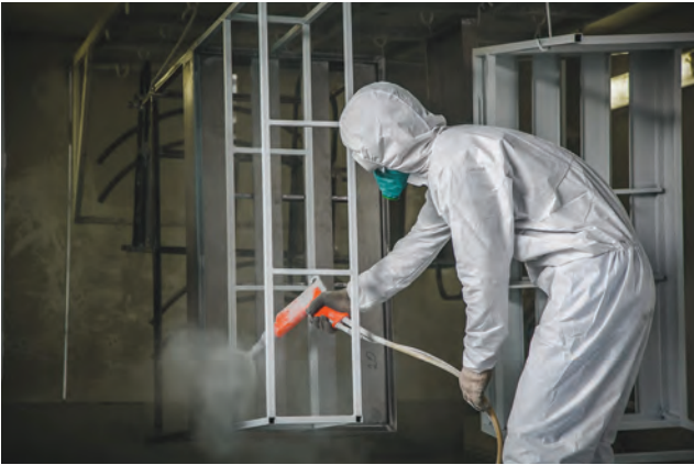
Figure 13.2 Paint spraying – risk of sensitising particularly if isocyanate based paint used and inadequate local exhaust ventilation
