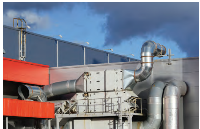
Figure 13.13(b) Large roof level system with access platform for maintenance of the filters and fans
