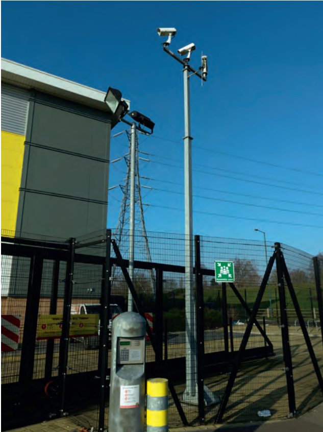
Figure 7.5 Security access and surveillance CCTV camera
