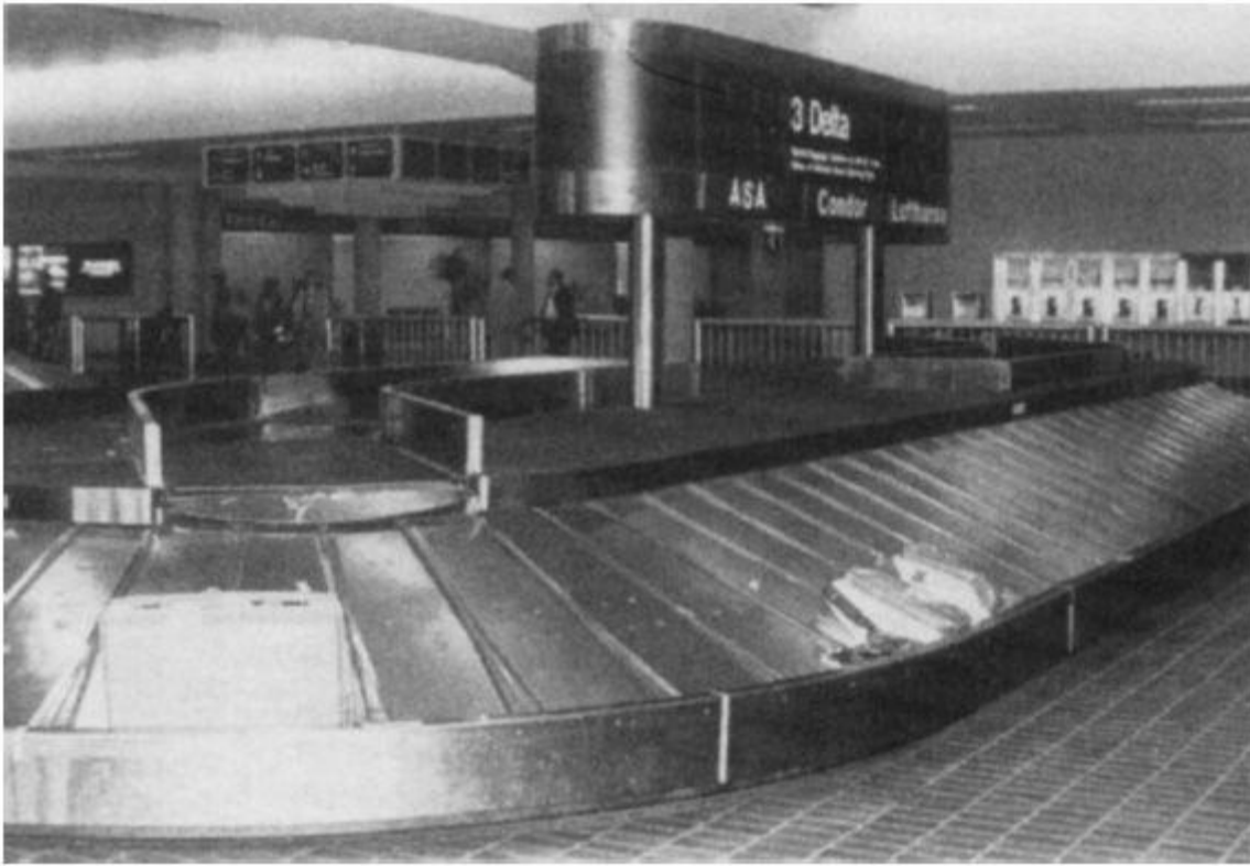
FIGURE 8.8 Designated baggage-delivery system.
