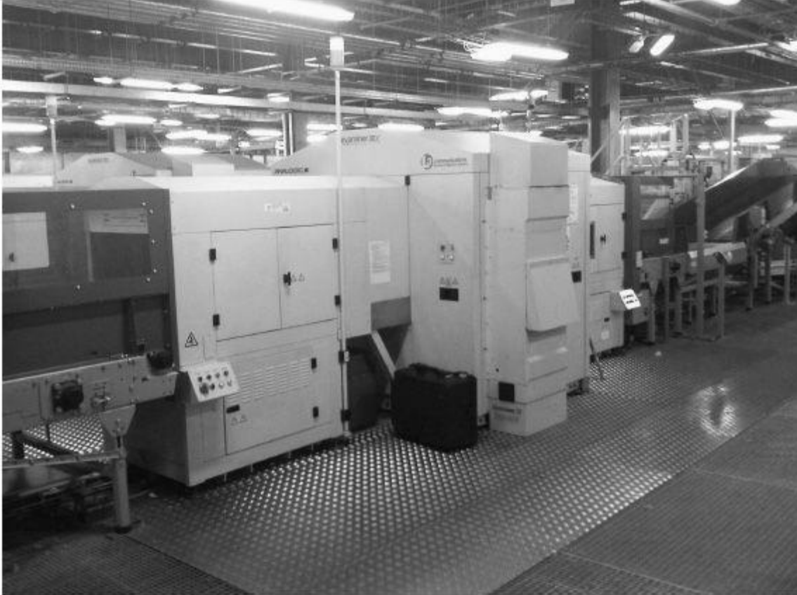
FIGURE 7.13 Hold-baggage screening equipment.
