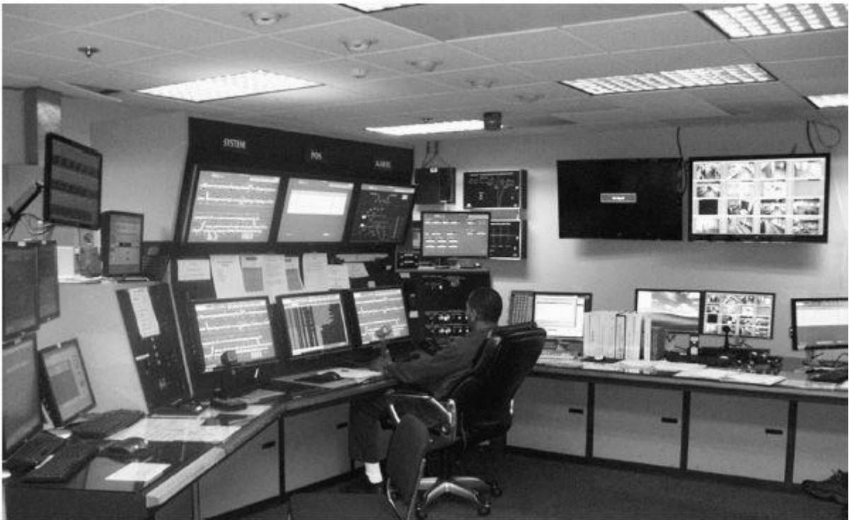
FIGURE 8.27 Control room for people mover at Atlanta Hartsfield-Jackson International Airport. (Source: Bombardier.)
