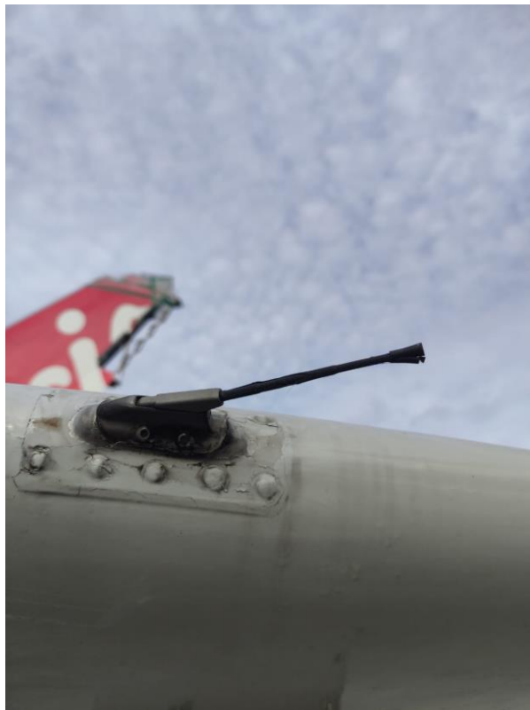
Gambar 4.5 Broken Static Discharge
