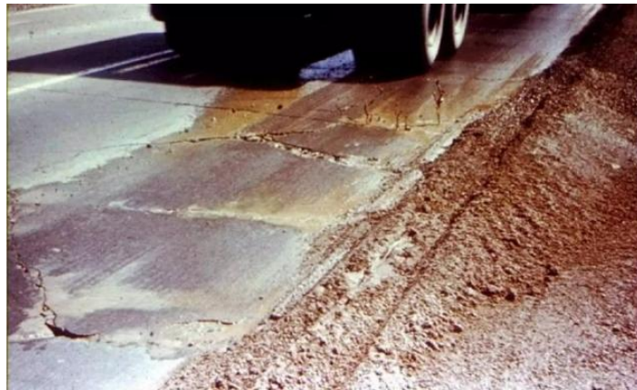
Gambar 3. 4 Merembesnya Air (Sumber: Slideshare.Net/Aguskerusakan-Perkerasan-Kaku )
