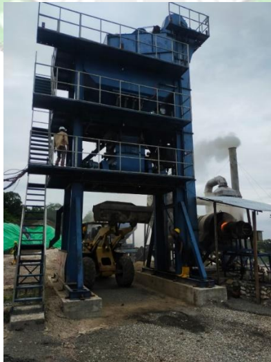
Gambar 4. 12 Asphalt Mixing Plant Sumber: Olahan Penulis, 2024
