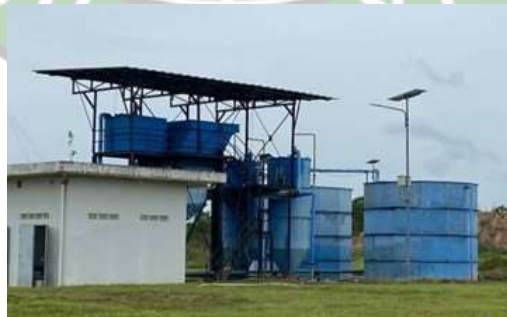
Gambar 4. 15 Water Treatment Plant (WTP) (Sumber : Dokumentasi Penulis, 2024)
