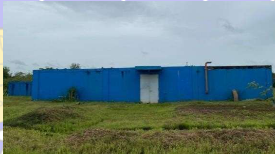
Gambar 4. 16 Water Treatment Plant (WTP) (Sumber : Dokumentasi Penulis, 2024)
