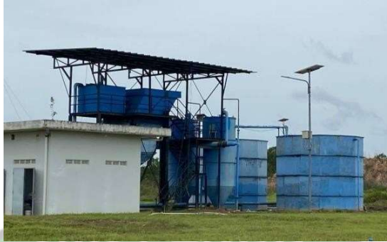
Gambar 4. 15 Ground Water Tank (GWT) (Sumber : Dokumentasi Penulis, 2024)
