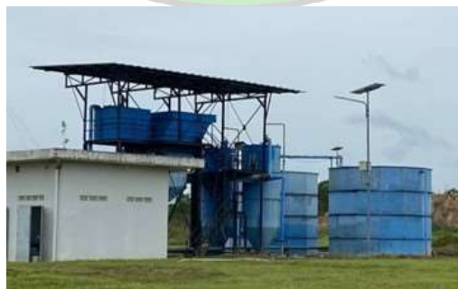
Gambar 4. 15 Water Treatment Plant (WTP) (Sumber : Dokumentasi Penulis, 2024)
