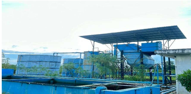
Gambar 4. 15 Ground Water Tank (GWT)
