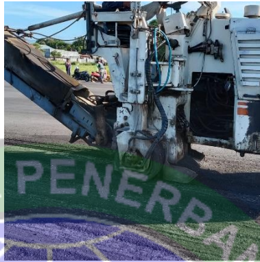
Gambar 4. 17 Pemotongan Aspal area Alligator Cracks
