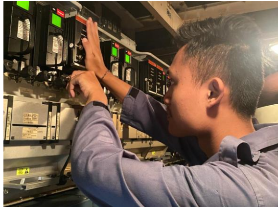
Gambar 4.12 Installation VHF 1 Transciever
