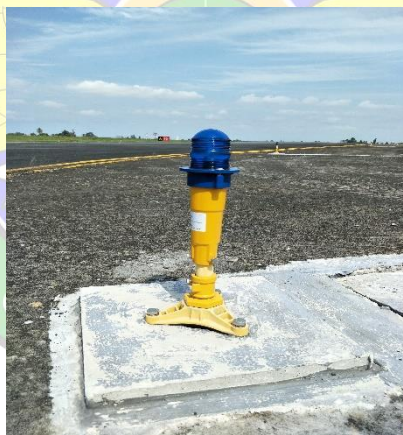
Gambar 2.30 Taxiway Edge Light
