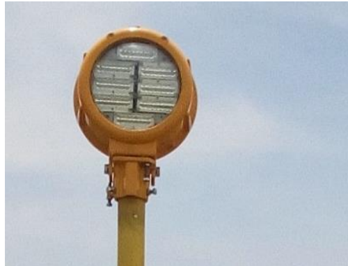
Gambar 2.20 Runway Threshold Identification Light (RTIL)
