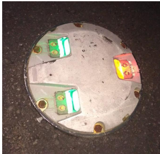
Gambar 4.2 Threshold Light Inset Green-Red
