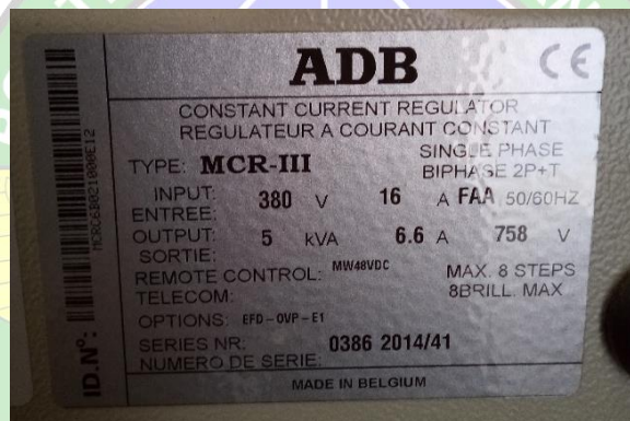
Gambar 2.13 CCR Taxiway Edge Light Rangkaian D
