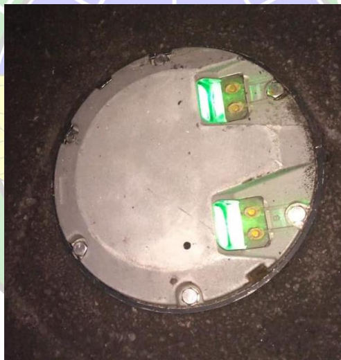
Gambar 4.3 Threshold Light Inset Green-Blank
