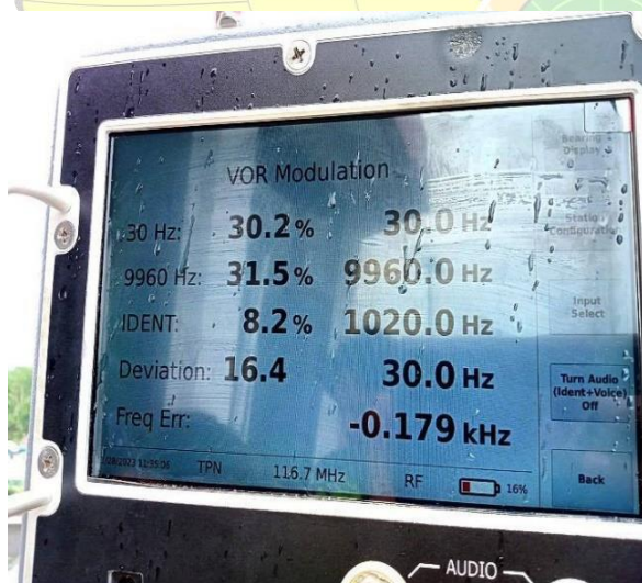
Ground Check DVOR
