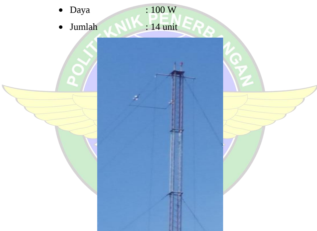
Gambar 2. 27 Obstruction Light Sumber : Bandara Internasional Juwata Tarakan
