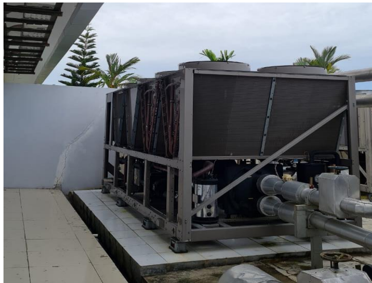
Gambar 2. 40 Chiller Double System Sumber : Bandara Internasional Juwata Tarakan
