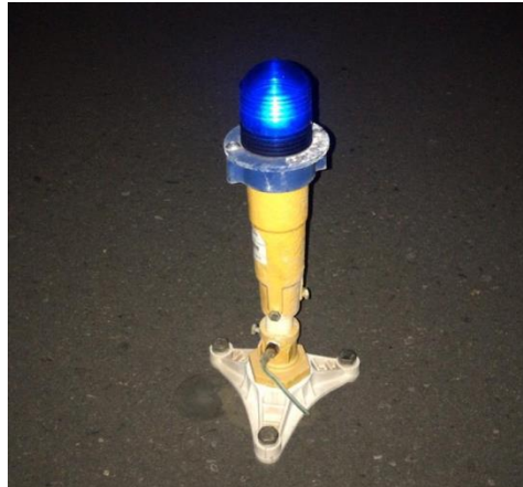
Gambar 2. 10 Taxiway Edge Lights
