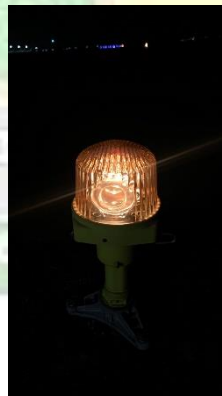
Gambar 2. 7 Runway Edge Lights
