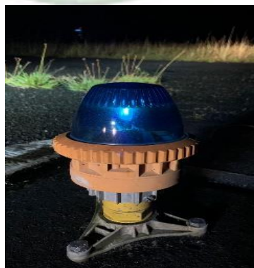
Gambar 2. 18 Turning Area Lights
