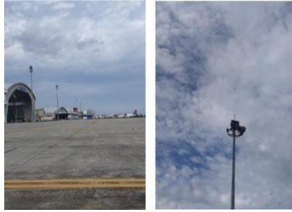
Gambar 2. 10 Apron Flood Light
