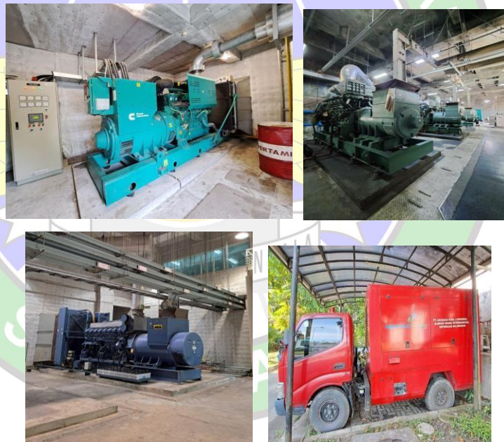
Gambar 2. 22 Genset MPH 1, MPH II, Genset gedung parkir, Genset Mobile
