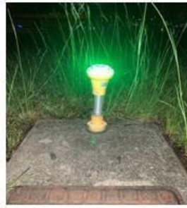
Gambar 2. 18 Heliport Perimeter Light
