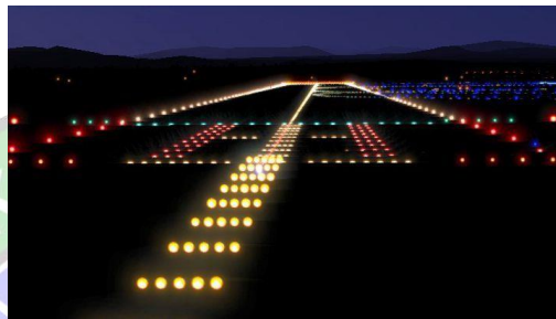
Gambar 3. 1 Airfield Lighting System
