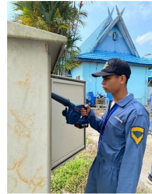
Maintenance Panel Floodlight
