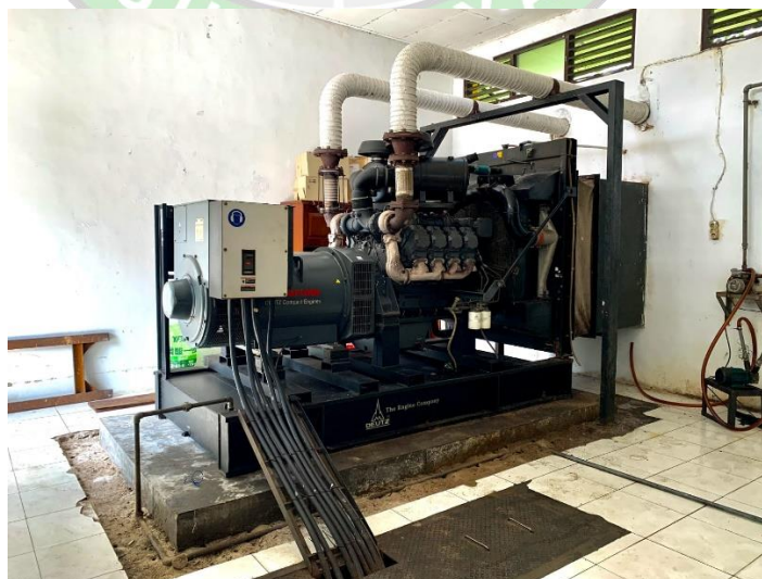
Gambar 2. 29 Generator Set 500 kVA
