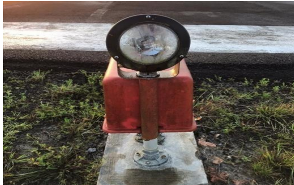
Gambar 2. 18 Runway Threshold Identification Light
