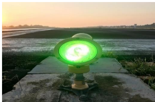
Gambar 2. 9 Lampu Threshold Elevated
