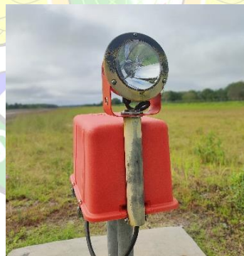
Gambar 2.24 Konstruksi Runway Threshold Identification Light Sumber: Bandara UPBU H. Asan Sampit
