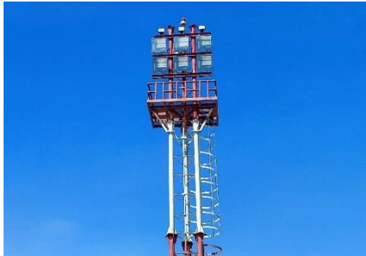
Gambar 2.29 Flood Light Sumber: Bandara UPBU H. Asan Sampit
