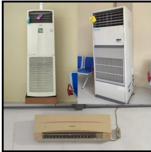
Gambar 2.11 Air Conditioning Sumber: Bandara UPBU H. Asan Sampit
