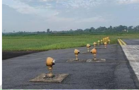
Gambar 2. 6 Runway End Light & Threshold
