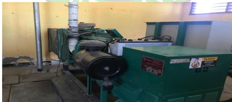
Gambar 2. 3 Generator Set 125 kVA
