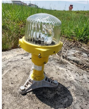
Gambar 2. 18 Runway Edge Light Elevated Sumber : Bandara Juwata Tarakan
