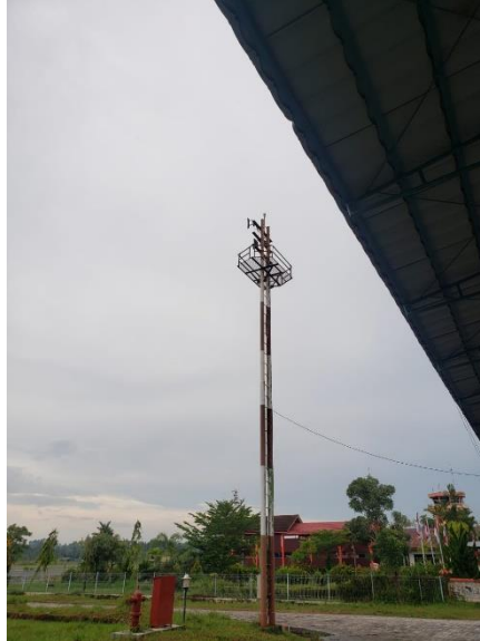
Gambar 2. 26 Flood Light Tiang Ganda
