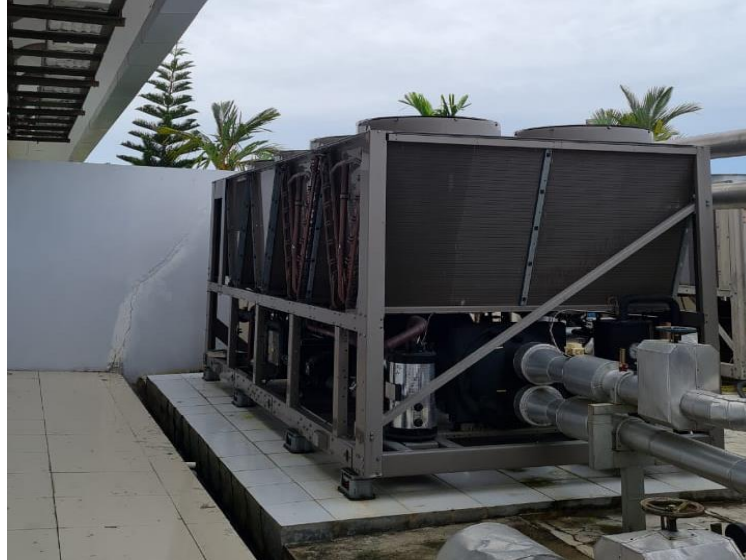
Gambar 2. 40 Chiller Double System Sumber : Bandara Juwata Tarakan
