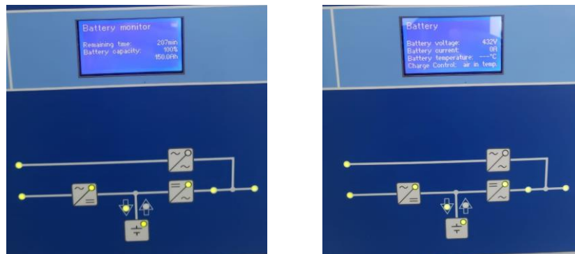
Gambar 4. 12 Monitoring performa battery Sumber : Bandara Juwata Tarakan
