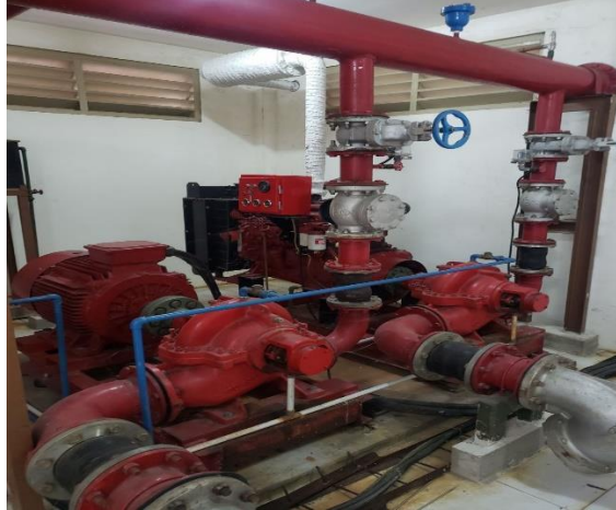
Gambar 2. 32 Pompa Hydrant Sumber : Bandara Juwata Tarakan
