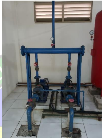
Gambar 2. 34 Pompa Transfer Sumber : Bandara Juwata Tarakan
