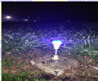
Gambar 2. 10 Taxiway Edge Light
