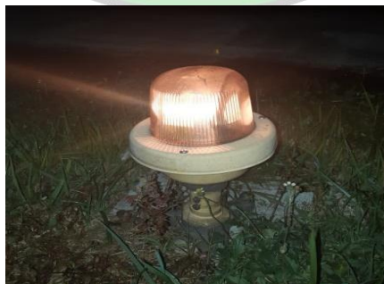
Gambar 2. 4 Runway Edge Light Elevated Sumber : Bandara Internasional Husein Sastranegara
