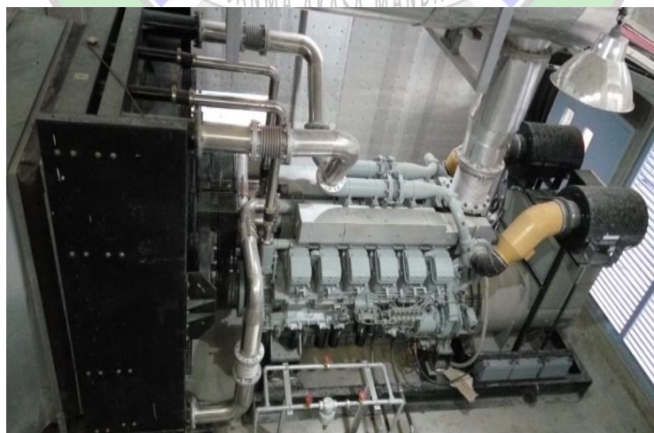
Gambar 2. 35 Generator Set 1500 KVA
