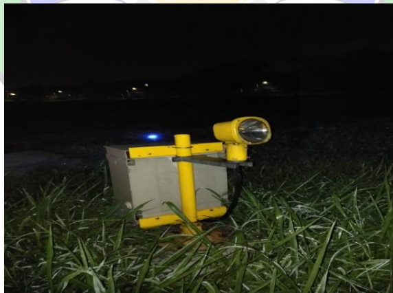
Gambar 2. 16 Runway Threshold Identification Light (RTIL)
