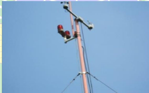
Gambar 2. 20 Obstruction Light Sumber : Bandara Internasional Husein Sastranegara
