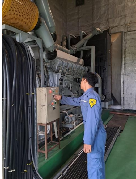
Gambar 5. 1 priming pum genset
