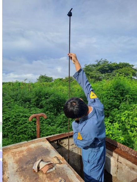
Gambar 5. 2 pengecekan ground tank BBM
