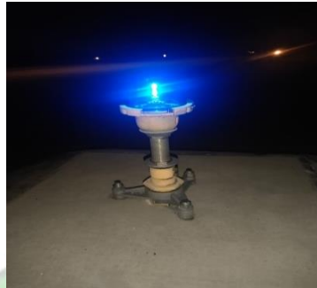
Gambar 2. 7 Taxiway Edge Light
