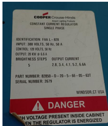
Gambar 3.5 Name Plate Constant Current Regulator Sumber: Bandara Internasional Sultan Hasanuddin Makassar
