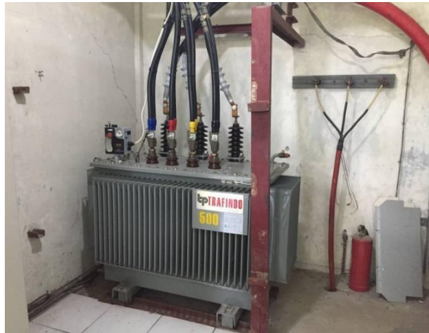
Gambar 2. 11 Transformator Step Down 500 Kva
