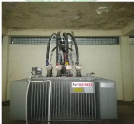
Gambar 2. 8 Transformator Step Up 1250 Kva
