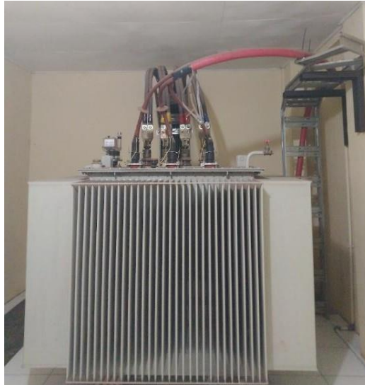
Gambar 2. 9 Transformator Step Up 1250 Kva
