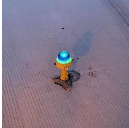
Gambar 2. 22 Taxiway Edge Light
