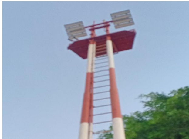
Gambar 2. 17 Apron Flood Light
