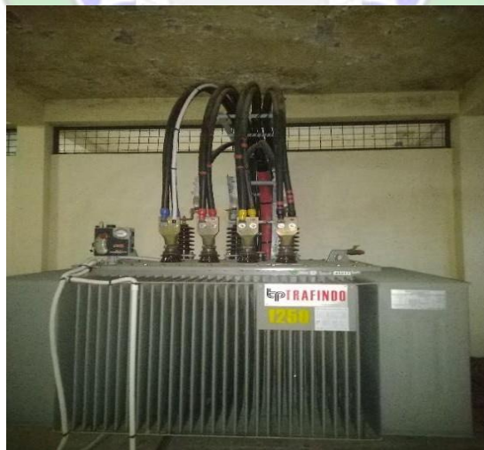
Gambar 2. 10 Transformator Step Down 500 Kva
