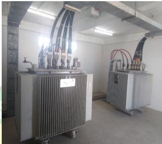
Gambar 2. 7 Transformator Step Down 1000 Kva
