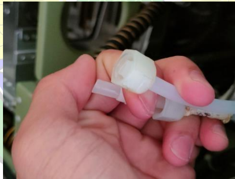
Gambar 4. 5 Leak on Pitot Line to GDC
