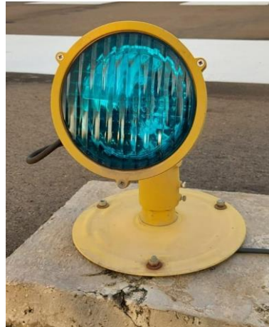
Gambar 2. 19 Runway Threshold Light
