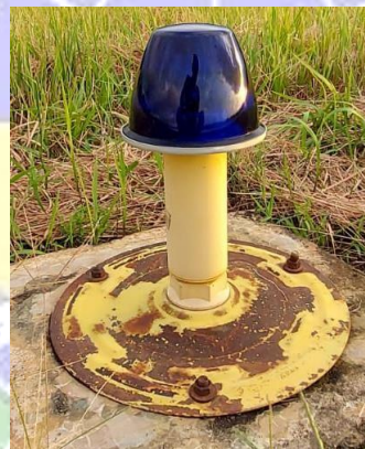
Gambar 2. 21 Taxiway Edge Light
