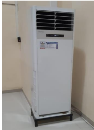
Gambar 2. 13 AC Floor Standing
