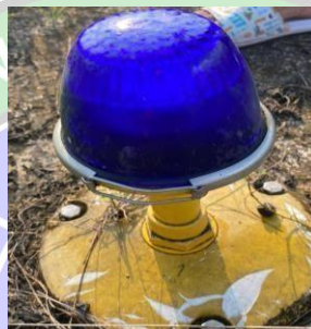
Gambar 2.26 Taxiway Edge Light Sumber : UPBU A.P.T. Pranoto Samarinda
