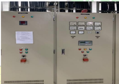
Genset Control Panel
