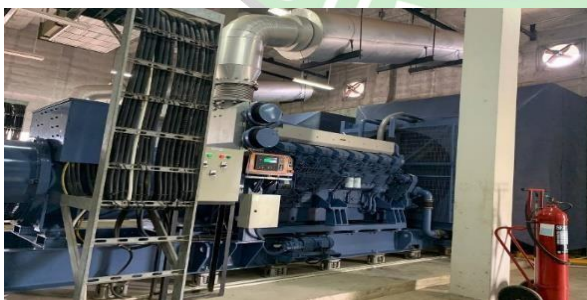
Genset (generator Set)
