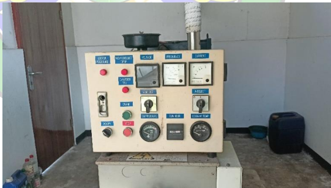
Gambar 2. 16 Generator Set 25 kVA
