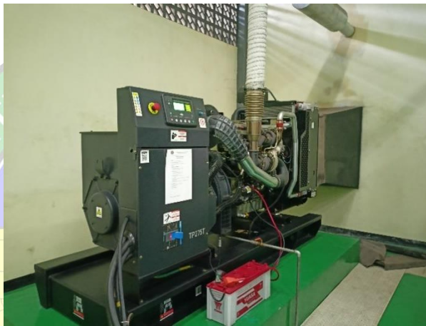
Gambar 2. 15 Generator Set 250 KVA
