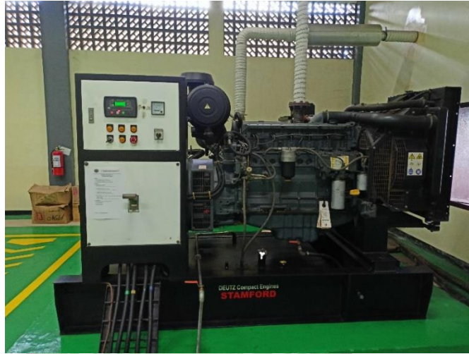
Gambar 2. 14 Generator Set 150 KVA
