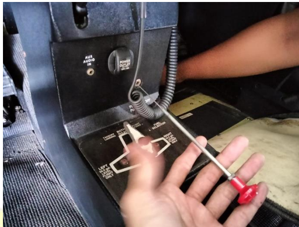
Gambar 4. 14 Fuel shutoff valve control cable terputus
