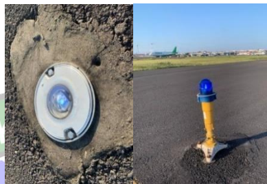
Gambar 2. 27 Lampu Taxiway Inset dan Lampu Taxiway Elevated
