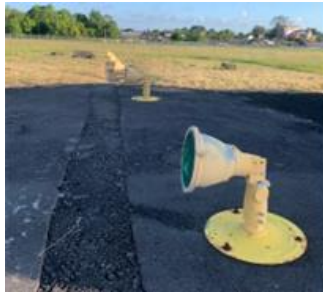
Gambar 2. 22 Lampu Threshold Elevated Unidirectional Sumber : Dokumentasi Penulis
