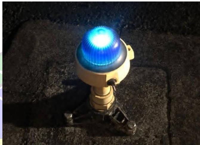
Gambar 2. 4 Taxiway Edge Light
