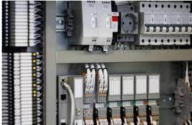
Gambar 3. 3 Progammmable Logic Control (PLC)
