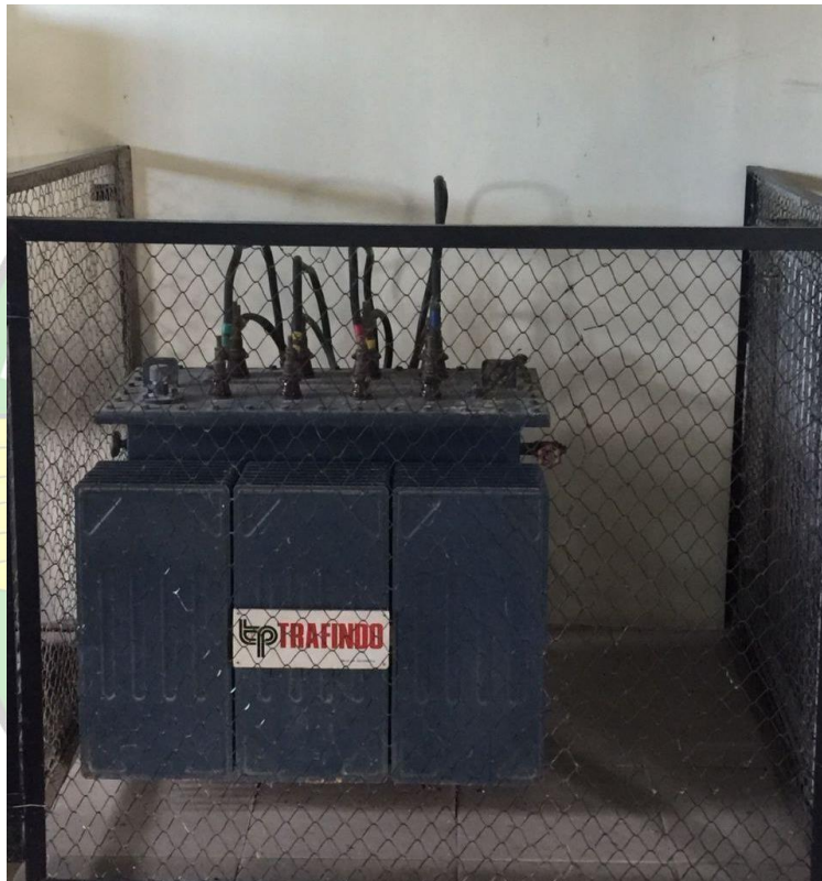
Gambar 2. 11 Transformator Step Up Genset
