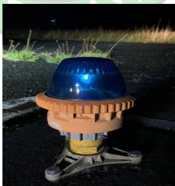
Gambar 2. 18 Turning Area Lights
