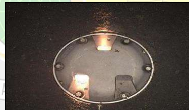
Gambar 4. 2 Inset Runway Edge Light
