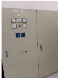
Gambar 4. 8 Panel Out Going Distribution Breaker
