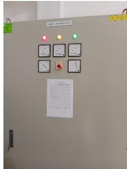
Gambar 4. 6 Panel Incoming PLN
