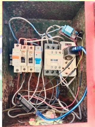
Gambar 4. 28 Instalasi Alat Kontrol Flood Light
