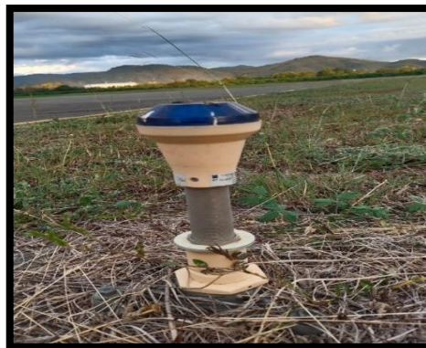
Gambar 2. 17 Taxiway Edge Light
