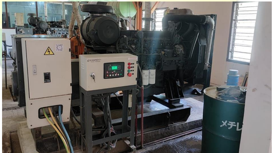
Gambar 4. 1 Genset STAMFORD 250 KVA
