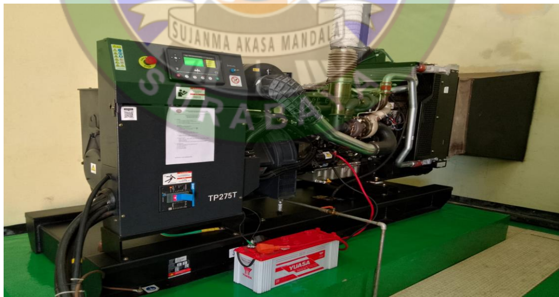
Gambar 2. 3 Generator set (Genset) Perkins 250 kVA
