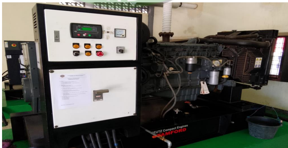
Gambar 2. 2 Generator set (Genset) Deutz 150 kVA
