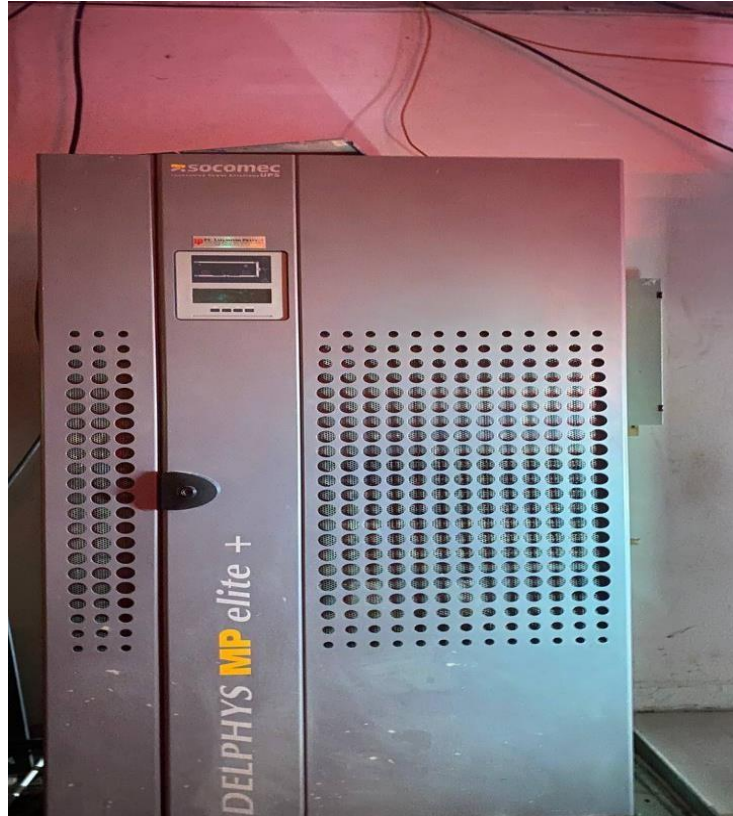
Gambar 4.9 UPS Socomec 120 Kva
