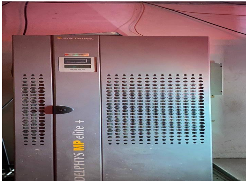
Gambar 3.4 UPS Socomec 120 Kva
