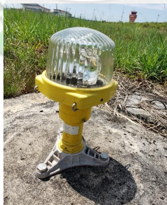
Gambar 2. 16 Runway Edge Light Elevated Sumber : Bandara Internasional Juwata Tarakan
