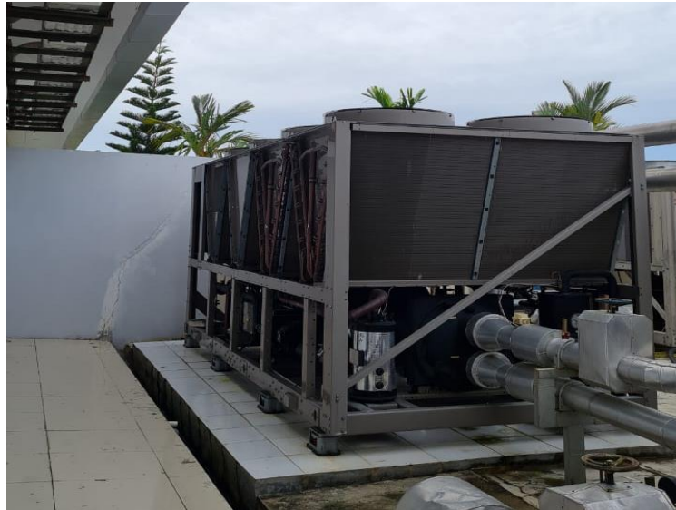
Gambar 2. 38 Chiller Double System Sumber : Bandara Internasional Juwata Tarakan
