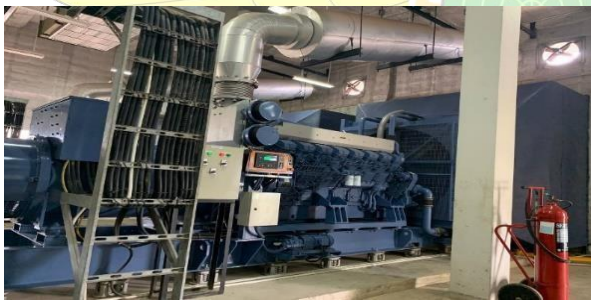
Genset (generator Set)
