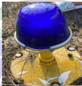
Gambar 2. Taxiway Edge Light Sumber : UPBU A.P.T. Pranoto Samarinda
