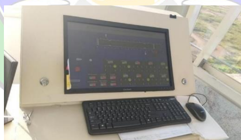
Gambar 2. 29 Panel Control Desk Sumber : UPBU A.P.T. Pranoto Samarinda
