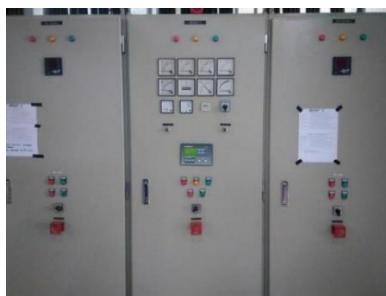
Gambar 2. 9 Genset Control Panel Sumber : UPBU A.P.T. Pranoto Samarinda
