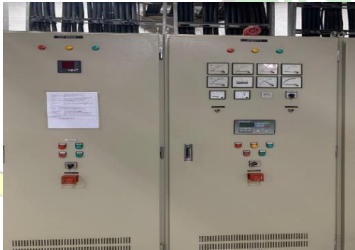
Genset Control Panel
