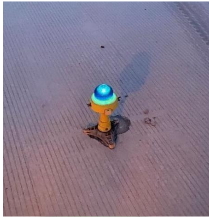
Gambar 2. 22 Taxiway Edge Light
