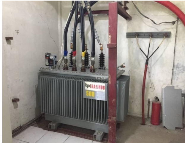
Gambar 2. 11 Transformator Step Down 500 Kva
