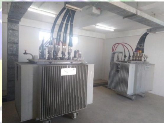
Gambar 2. 7 Transformator Step Down 1000 kVA
