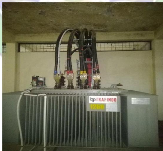
Gambar 2. 10 Transformator Step Down 500 Kva
