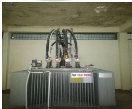
Gambar 2. 8 Transformator Step Up 1250 Kva
