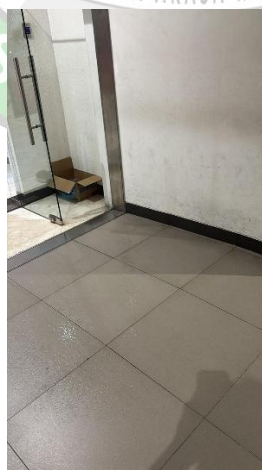
Gambar 14 Monitoring kebocoran saat hujan di area koridor Terminal 1
