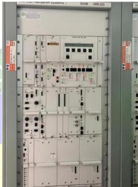
Gambar 3. 11 Transmitter DVOR Merk InterScan
