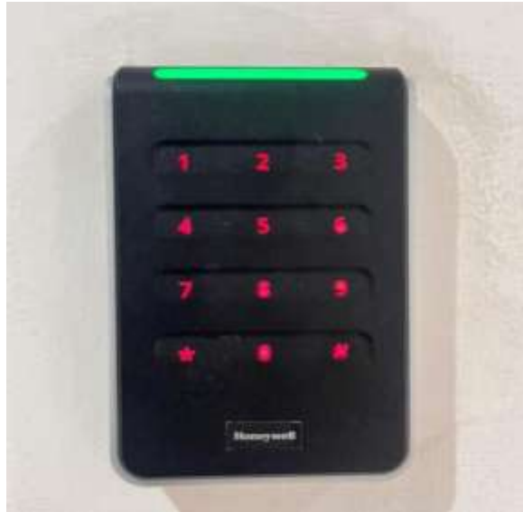
Gambar 3. 7 Access Door Control 1
